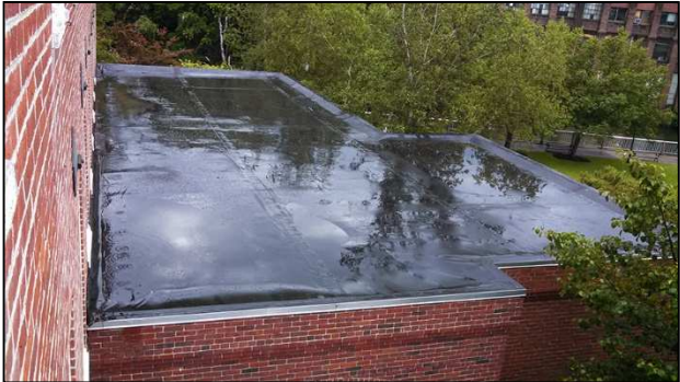
Figure 10: Looking down onto the Power House roof, with large areas of water pooling.
