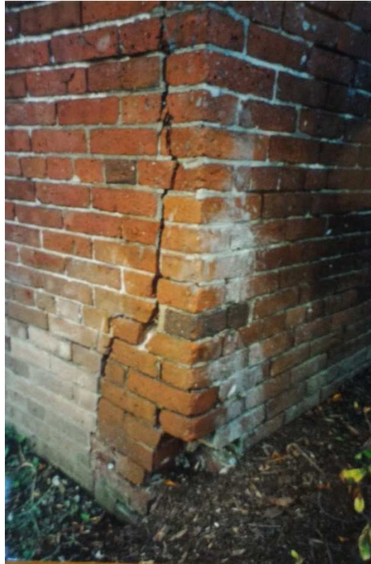
Figure 17: Masonry damage to Belknap Mill following January 2000.
