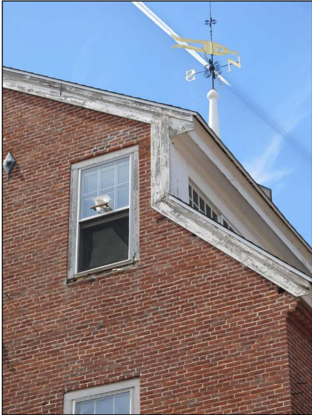
Figure 9: Peeling Paint at eaves/soffits
