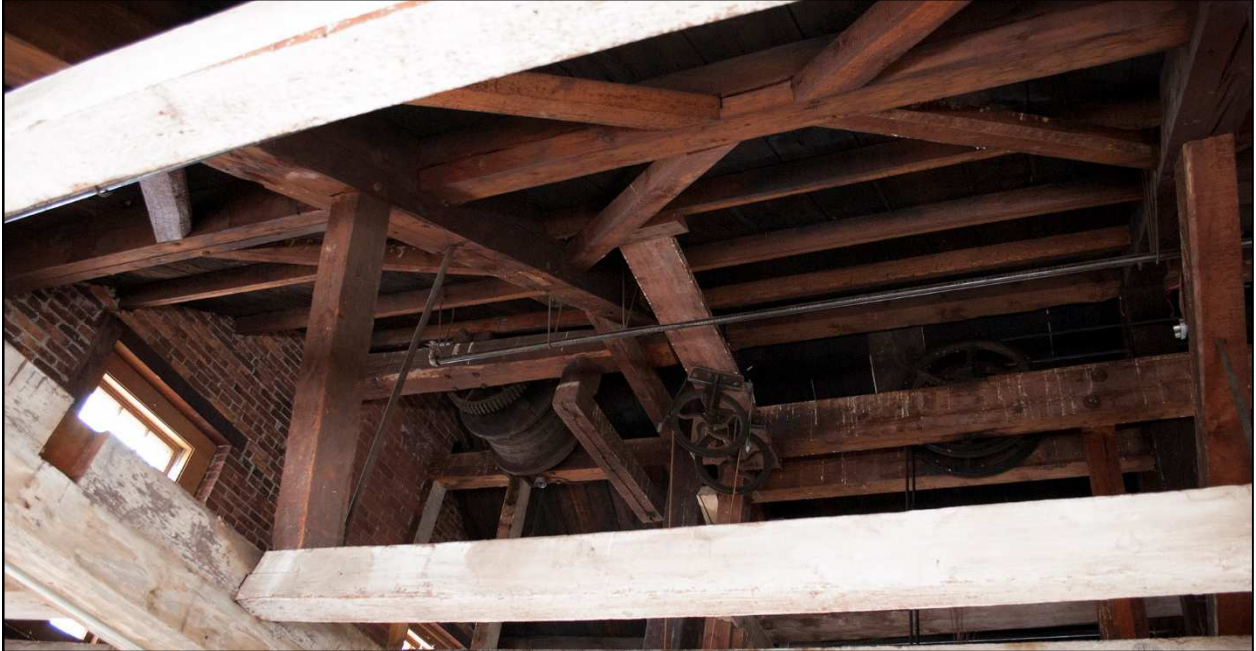
Figure 16: Elevator mechanisms, Belknap Mill attic.
