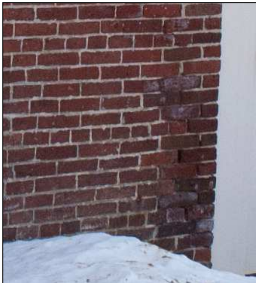
Figure 3: Mortar loss near the entrance door.
