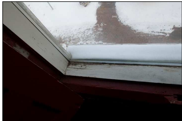
Figure 25: Rotten sill, stair tower
