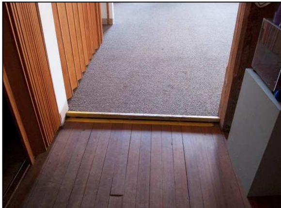
Figure 15: Transition of floor from gallery to knitting room, first floor Belknap Mill
