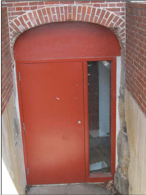
Figure 7: Basement door with cracked sidelight
