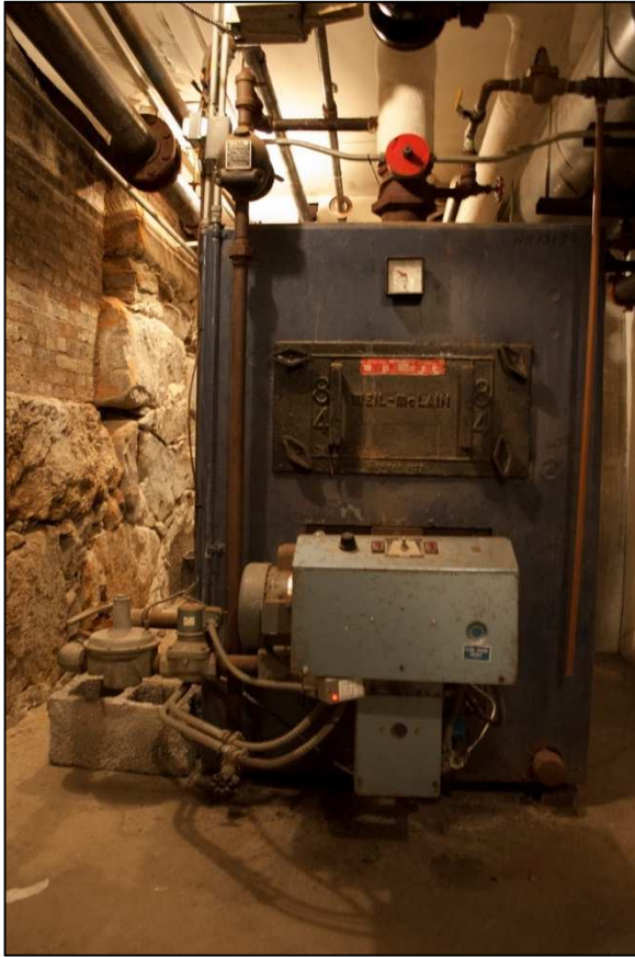
Figure 13: Belknap Mill boiler
